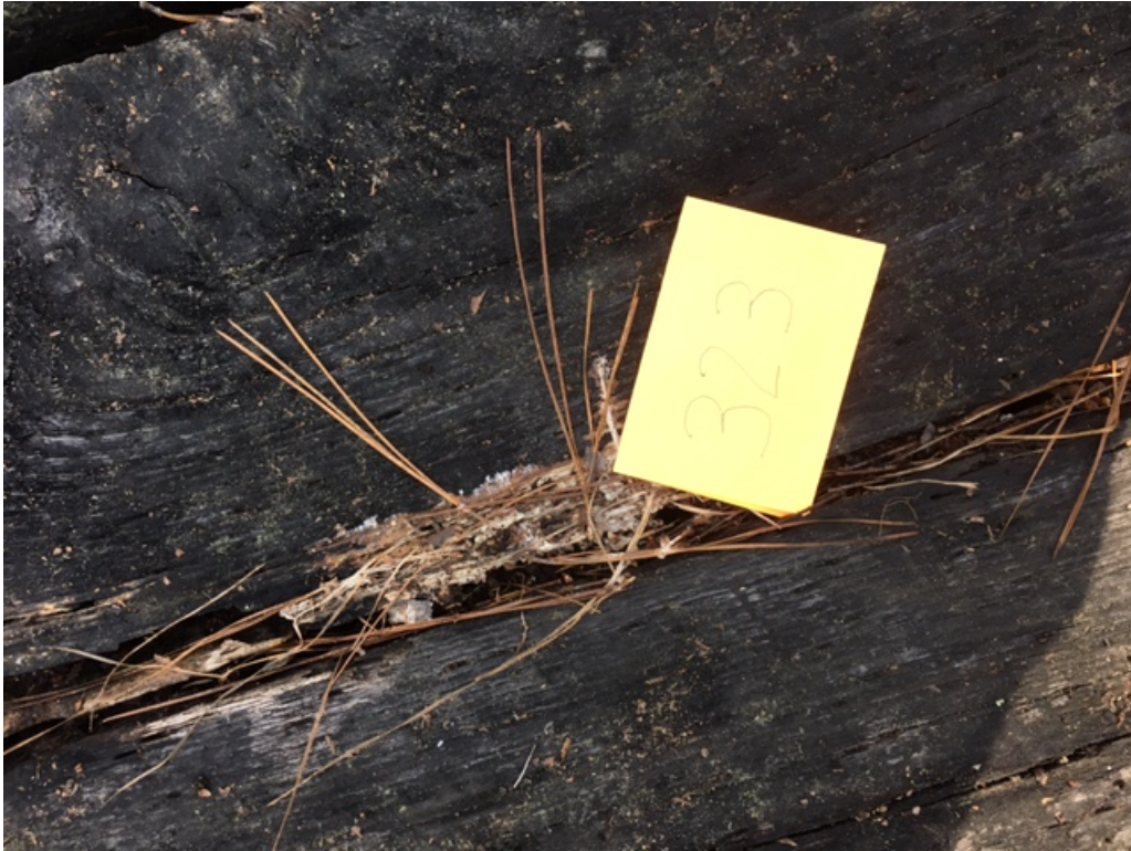
Figure 3 - Tie #323 showing decay damage.
