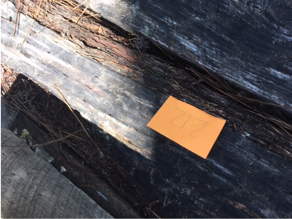
Figure 5 - Tie #212 with decay.
