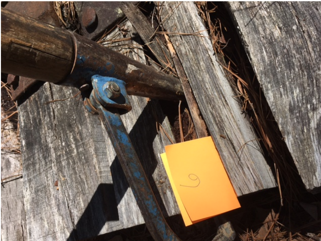
Figure 4 - Tie #6 with heavy decay.
