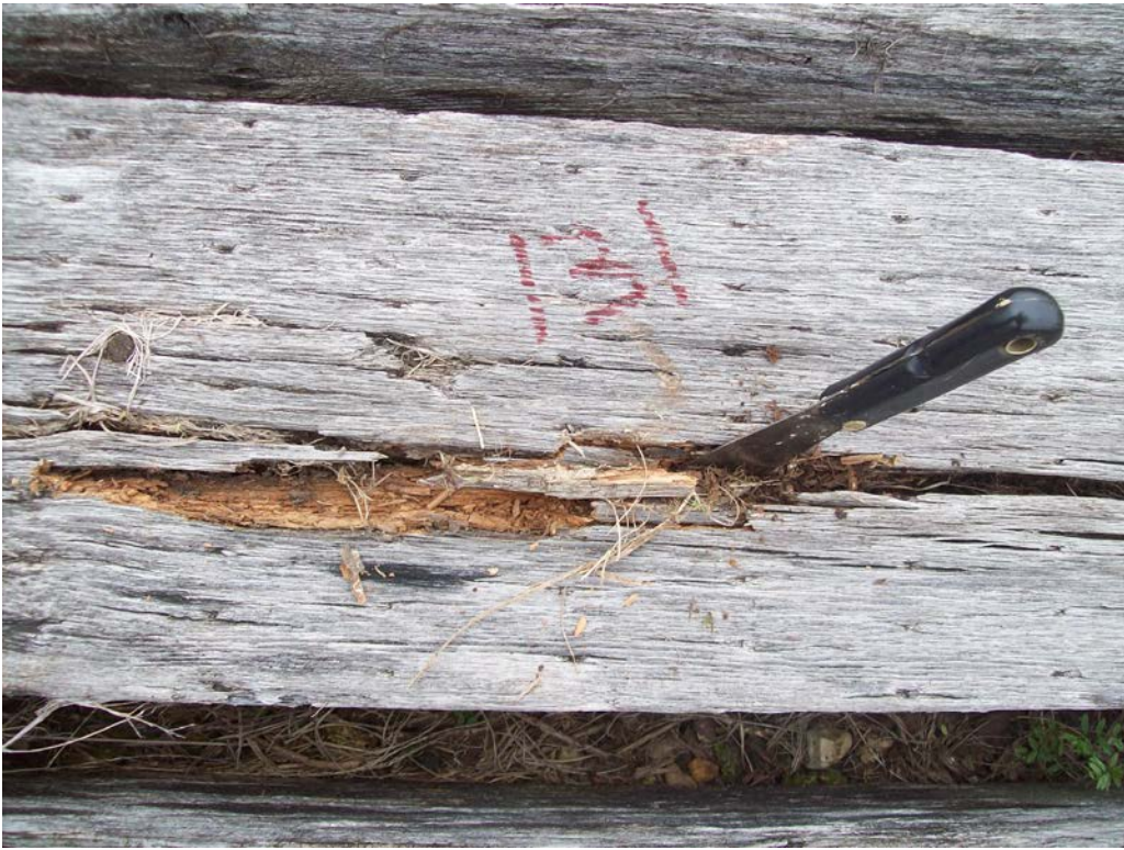
Figure 7 - Tie #131 with decay.
