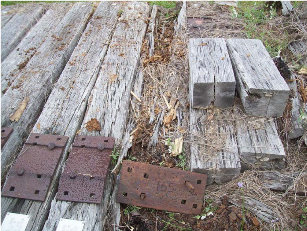
Figure 8 – Tie #165 failed due extensive decay.
